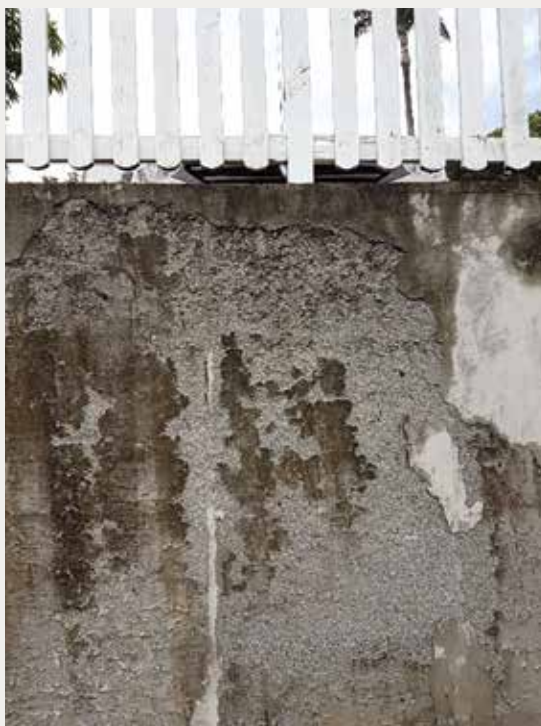
Peeling on the surface of a retaining wall © Loïc Divet
